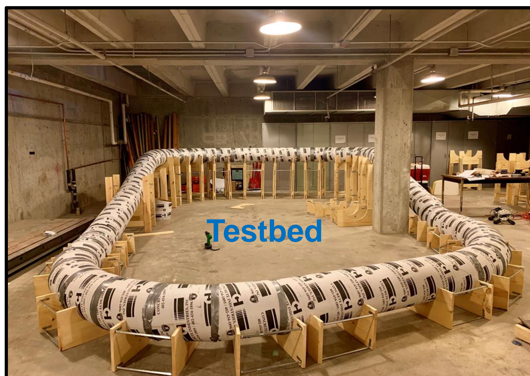
Figure 3. simulated pipeline plant with 14" diameter pipe.
